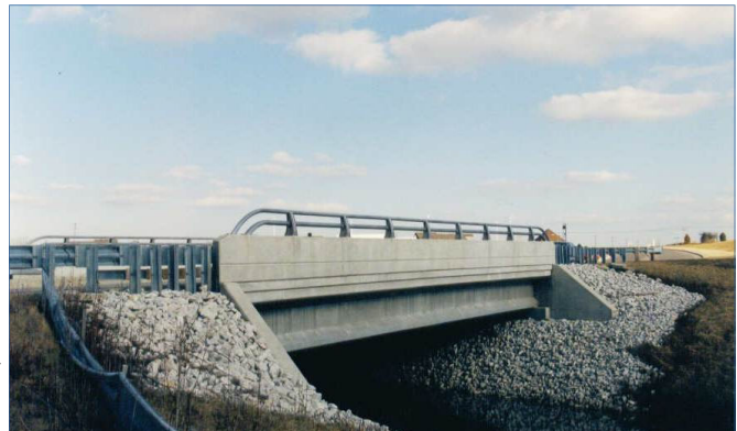
Ridge Road Bridge over the Waubensee Creek Design and Construction Phase by Rempe-Sharpe
