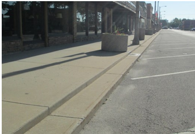
ADA Compliance Concerns
