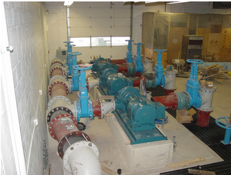
Addressed with Pumping Station to Create Uniform Pressure
